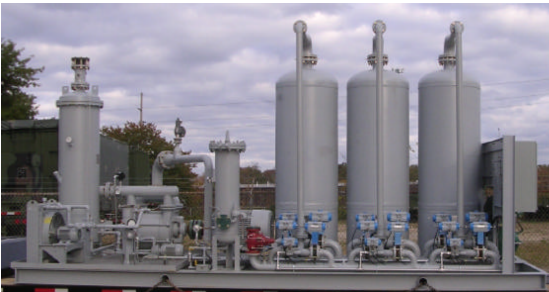
Figure 6. A SPEC plant used to treat smaller flows
